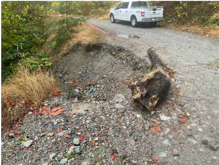
Erosion at downstream right bank
