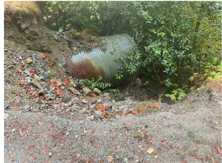
Erosion downstream right bank
