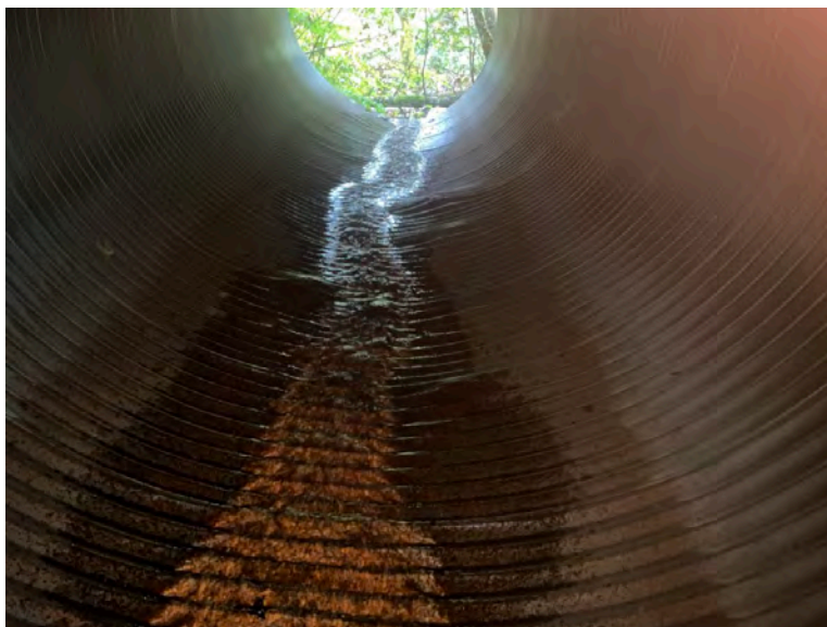
Damage along the floor
