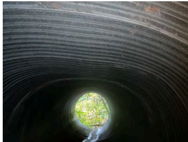
Damage along roof
